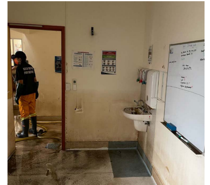
Water Level in CTI clinic room
